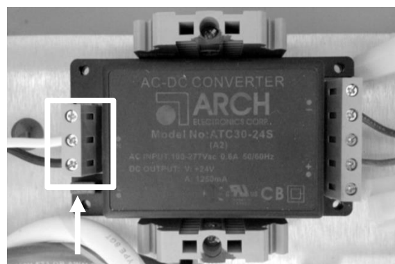
Picture 3 – AC Control Power Terminals
