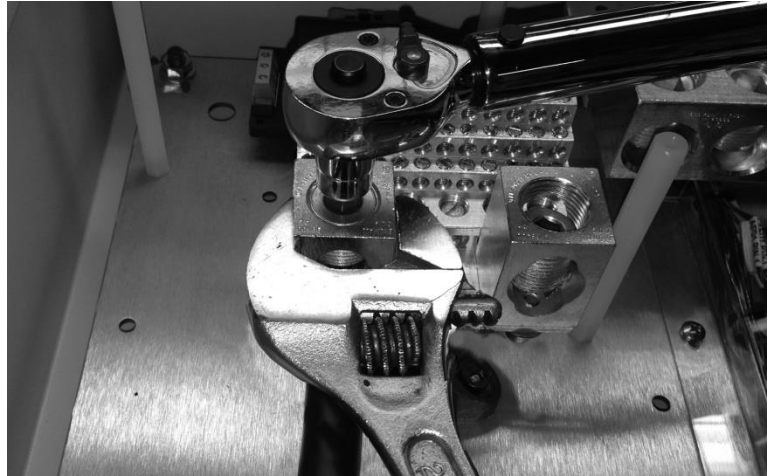
Picture 1 – Output Lug with Backup Wrench
